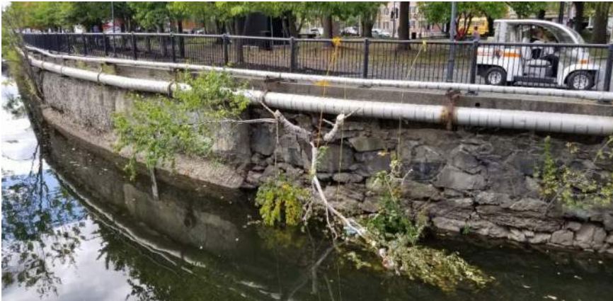
Polygon No.: 90 Photo No.: CV_Poly10a Date: 9/25/2019 Direction Photo Taken: Southwesterly Description: The vegetation growing out of canal wall is a 3-trunked tree of heaven tree at approximately 4 inches diameter at breast height. A recently cut birch tree tied with rope was also observed along the canal wall.
