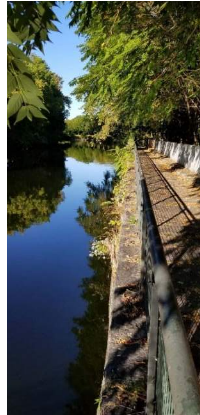
Polygon No.: 78 Photo No.: 78 Date: 9/27/2019 Direction of Photo Taken: Westerly Description: Vegetation growing out of the canal walls include tree of heaven and mulberry and herbaceous species such as purple loosestrife and mullein.
