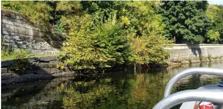
Polygon No.: 69 Photo No.: 69 Date: 9/26/2019 Direction Photo Taken: Northwesterly Description: The trees growing out of canal wall include tree of heaven and elms at approximately 10 feet tall.
