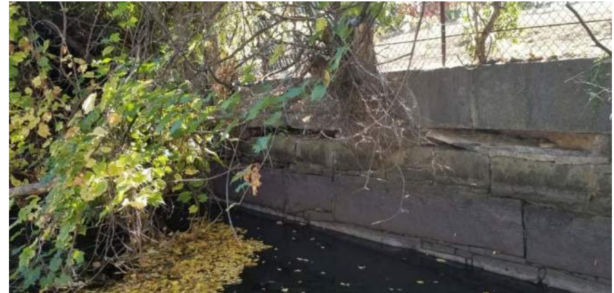
Polygon No.: 57 Photo No.: 57 Date: 9/26/2019 Direction Photo Taken: Easterly Description: Vegetation growing out of the canal wall includes ash trees at approximately 6 to 8 inches diameter at breast height.
