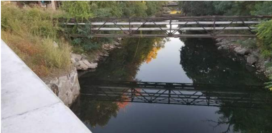
Photo Location No.: P-2 Date: 9/25/2019 Direction Photo Taken: Southwesterly Description: Vegetation is growing on the riprap shoreline along both sides of the canal.
