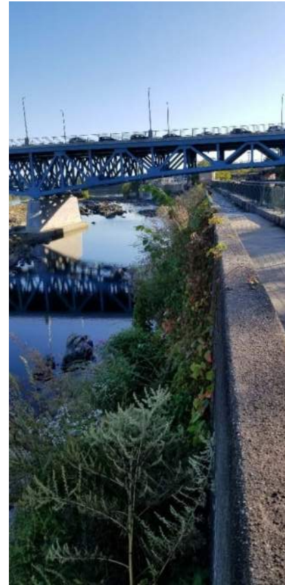
Polygon No.: 75 Photo No.: 75a Date: 9/27/2019 Direction: Northeasterly Description: Vegetation is growing from small sill under the first block down on the canal wall and is dominated by herbaceous plants such as ragweed, purple loosestrife, aster, scattered ferns, golden rod spp., scattered mulberry, elms, and buckthorn.
