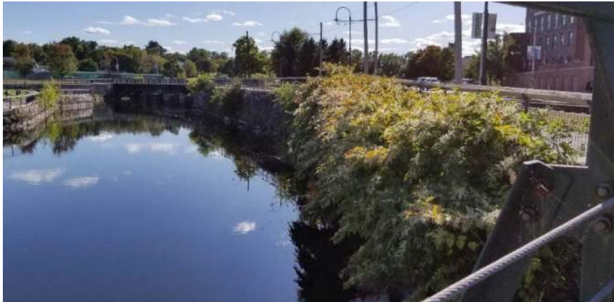
Polygon No.: 18 Photo No.: 18 Date: 9/25/2019 Direction Photo Taken: Southwesterly Description: Approximately 20 percent of the canal wall has woody trees, shrubs, and/or herbaceous plants growing on it. The vegetation includes tree of heaven, maple, common mullein, Japanese knot weed, and ragweed. Japanese knot weed coverage increases with closer proximity to the National Park Service boat dock.
