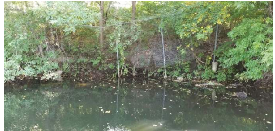
Photo Location No.: P-4 Photo No.: P-15 Date: 9/26/2019 Direction Photo Taken: Easterly Description: Dense vegetation is growing on earthen banks along the canal.
