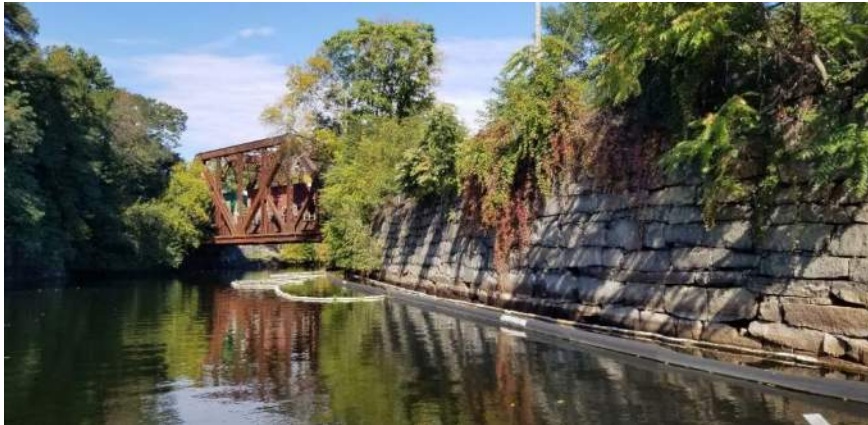
Polygon No.: 66 Photo No.: 66a Date: 9/26/2019 Direction Photo Taken: Northerly Description: The vegetation growing out of the eastern side of the canal wall (right side of the photograph), at the top of the wall, includes trees, such as tree of heaven and birch, and vines, such as Boston ivy.
