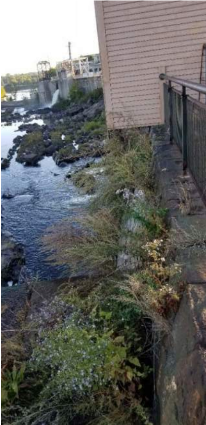
Polygon No.: 74 Photo No.: 74 Date: 9/27/2019 Direction: Northeasterly Description: Ragweed is growing out of the canal wall located beneath the building.
