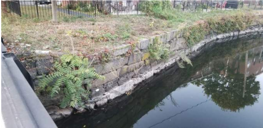
Polygon No.: 39 Photo No.: 39 Date: 9/25/2019 Direction Photo Taken: Northerly Description: A few small tree of heaven trees are growing out of the canal wall, near the top of the wall.
