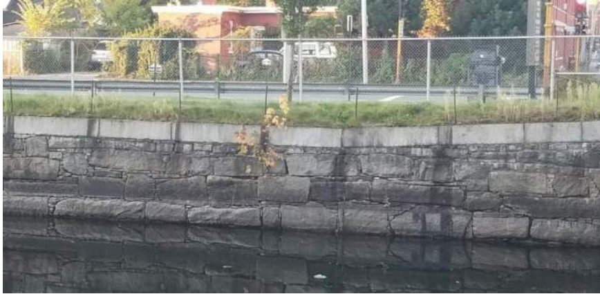
Vegetation Point No.: VP-10 Photo No.: VP-13 Date: 9/26/2019 Direction Photo Taken: Southerly Description: A small maple is growing out of the canal wall, near the top of the wall.
