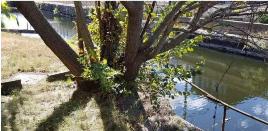
Polygon No.: 13 Photo No.: 13 Date: 9/25/2019 Direction Photo Taken: Southerly Description: There is one elm tree and one mulberry growing out of concrete portion of the canal wall.
